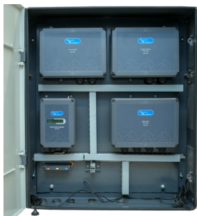
Interior View of xMasm10 - Wired Solution
