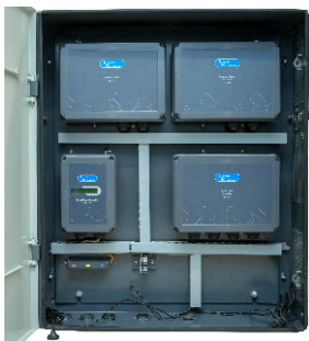
Interior View of xMasm10 - Wired Solution
